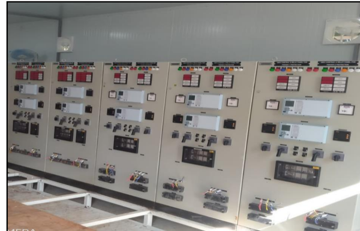
CRP installation for SCADA
