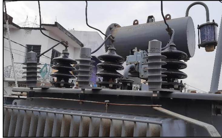
LA replacement of DTR
