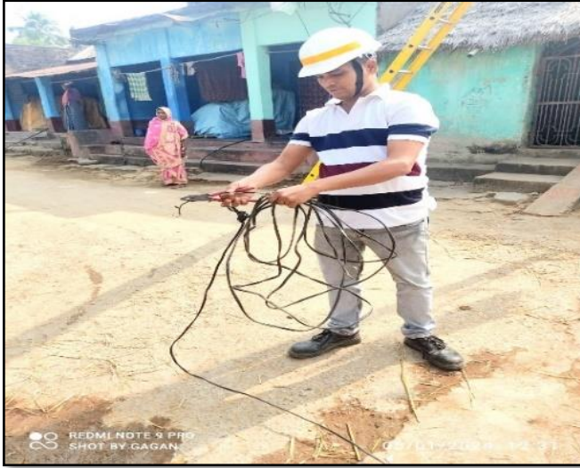
Illegal Hooking Removal
