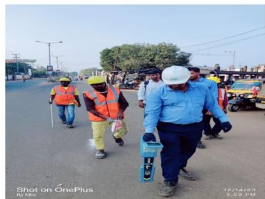
Cable route tracing before excavation near cable route to avoid external damage
