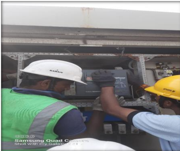
ACB replacement in CSS
