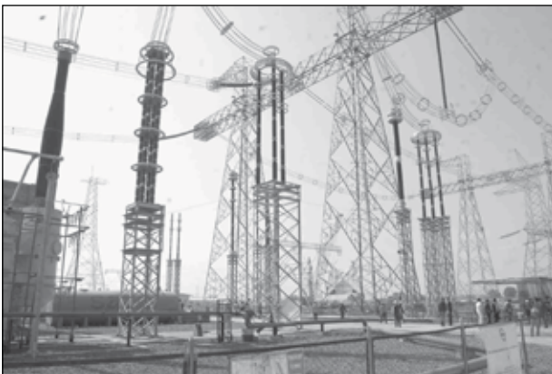
Fig: 1200kV (World's Highest Voltage level) bay at the National Test Station
